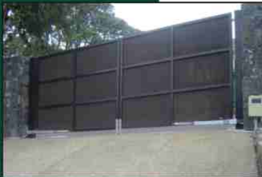
Steel framed hinged gates
